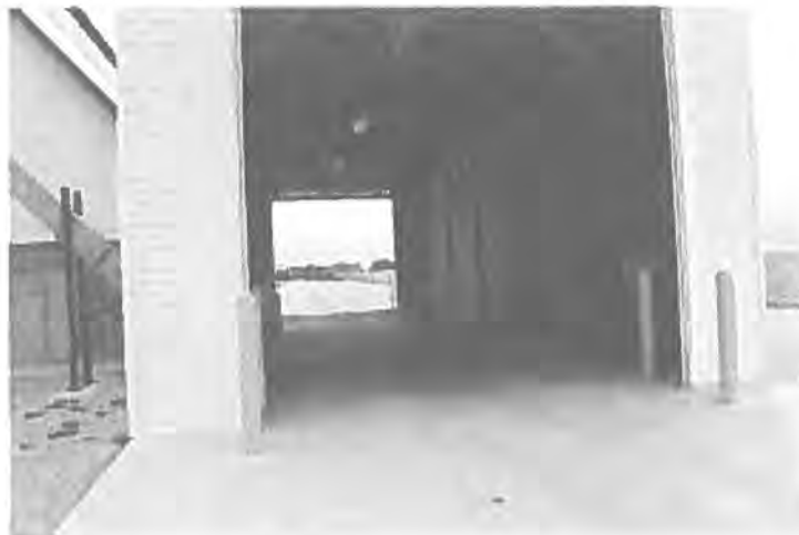
View of what the future tractor trailer unloading building (OC-2) adjacent to dry fertilizer building will look like when completed
